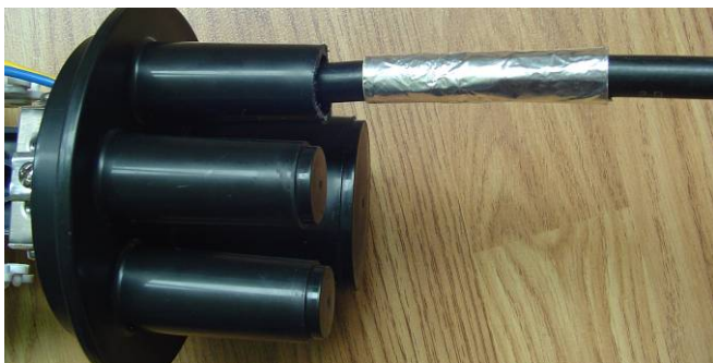
(12) Bound and even the heat-shrink part with aluminum paper to avoid burn caused by high temperature of blast burner.
