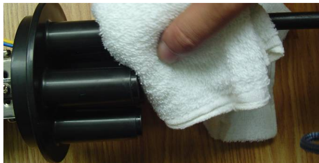
(10) Sealing of cable and base: clean the entry ports and cable with 10cm long by scrubber.
